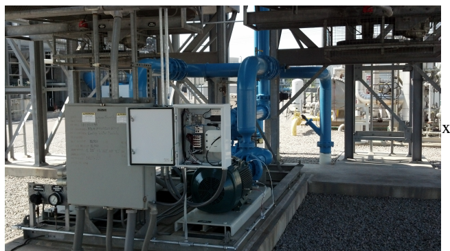
Fig: 1 NI CompactRIO system connecting plant-wide assets for a machine condition monitoring solution at Duke Energy
